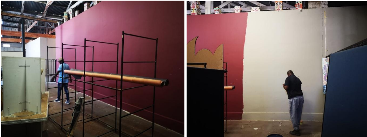
Above: The walls being painted at our new office space in the KWV Building, Montagu.
